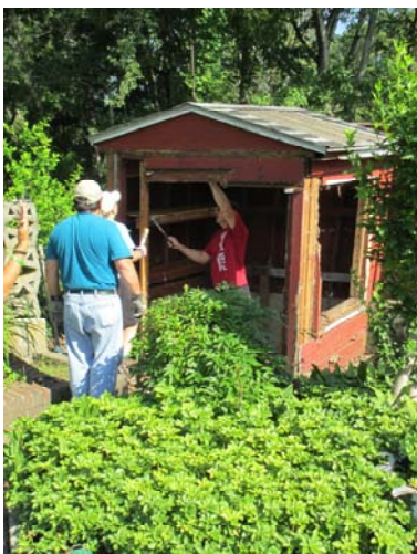
More than 9,000 volunteers have helped with demolition and rebuilding homes impacted by Hurricane Sandy. Most have been engaged with VOAD partners Rebuilding Together Bergen County and Habitat for Humanity Bergen County.
